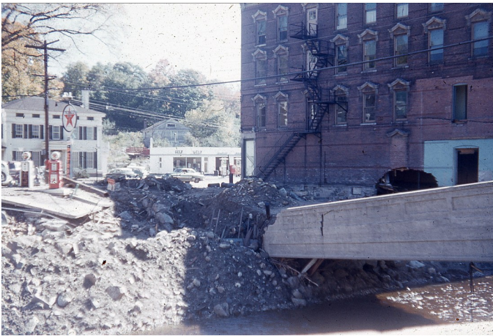
The washed-out remains of the bridge at the bottom of Lake Street
